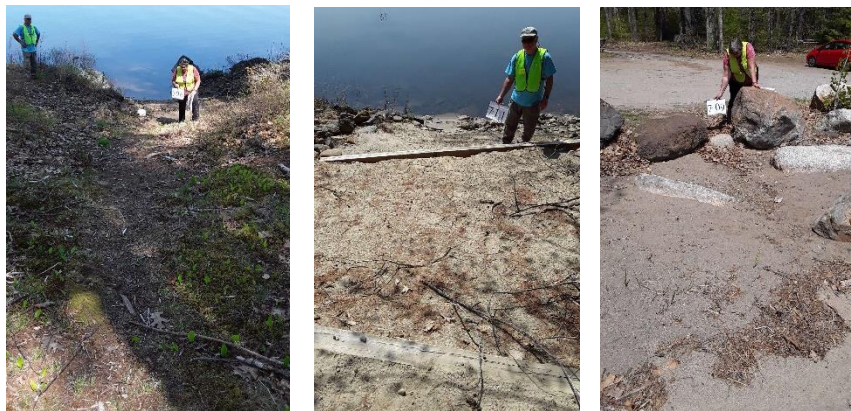
Example sites identified in the Stinchfield Beach neighborhood in Sector 7: Site 7-06 (left) erosion on a shorefront pathway, site 7-11 (middle) unstable soils on a steep slope, and site 7-09 (right) runoff from a town parking lot is creating a channel with flow to Androscoggin Lake.
