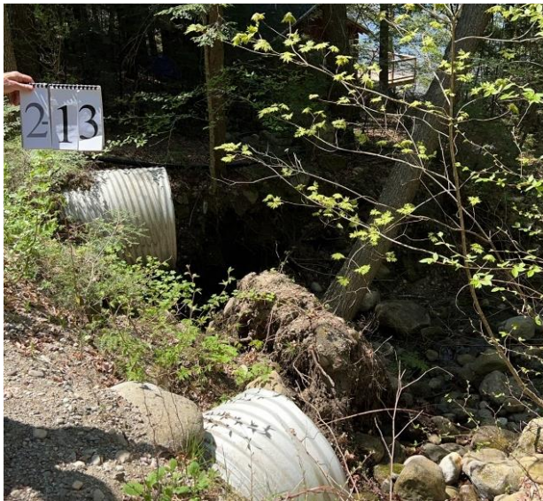
Bank failure at a culvert outlet (site 2-13) on Holman Terrace in Sector 2.
