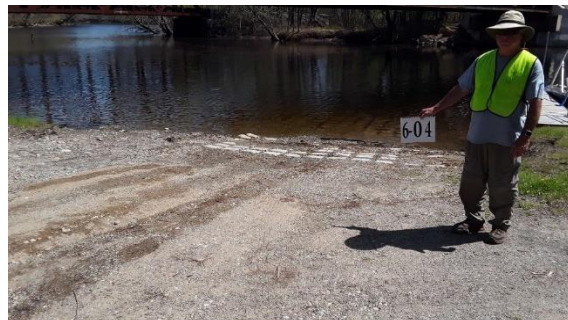
Erosion documented at a commercial boat launch in Sector 6 (site 6-04).
