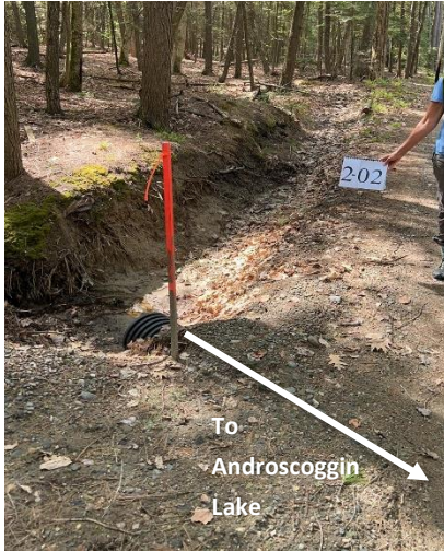
Ditch, culvert, and road surface erosion identified on a private gravel road that drains to Androscoggin Lake.
